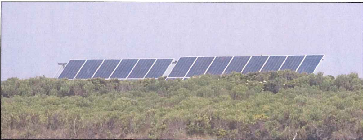
Figure 7: Photovoltaic Ground Array
